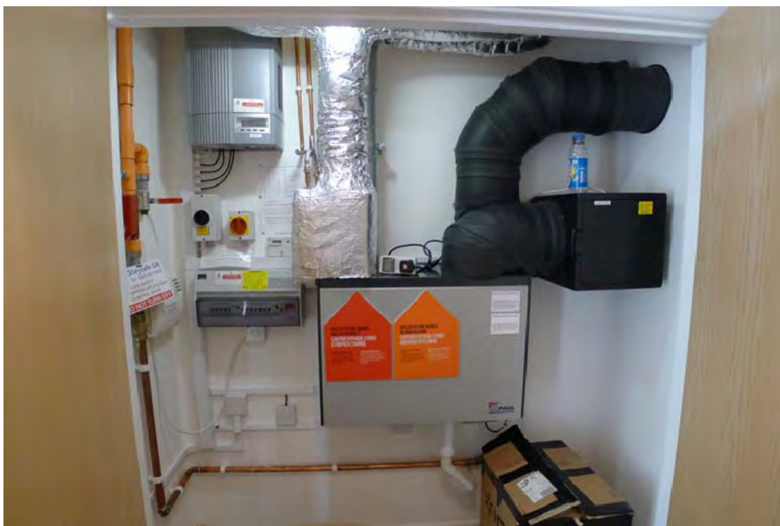
Figure 2-12. Ventilation system in the Larch House. A heater battery is installed directly above the ventilation unit (wrapped in silver foil) and this is supplied with hot water from the central heating boiler. The heater battery is on the left with foil covered insulation, the intake and exhaust ducts are on the right and insulated with vapour impermeable Armaflex insulation. The frost heater and pre-filter are in the black insulated box on the right.
