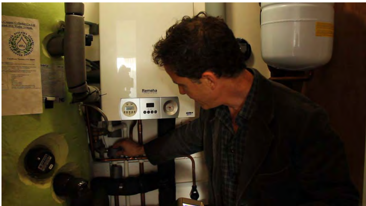
Figure 4-1. Justin Bere from bere:architects explaining why the pipe insulation needed to be improved.
