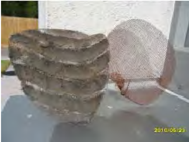
Figure 7-1. Intake and exhaust mesh, showing accumulated debris from neighbouring construction site.
