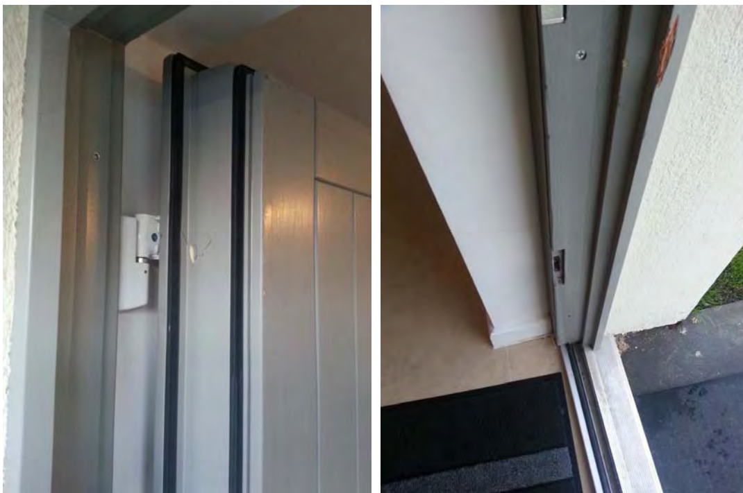
Figure 8-6. Lime house front door damages in December 2012
