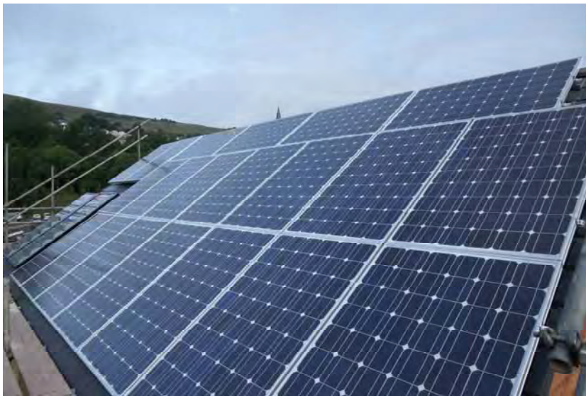
Figure 2-15. PV array at the Larch House
